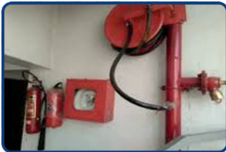
Fire Hosebox, hose reel & Accessories work
