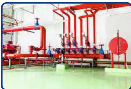
Trunkey Projects of fire Fighting systems
